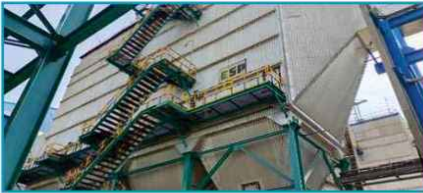
Performance Evaluation of ESP attached to Boiler
