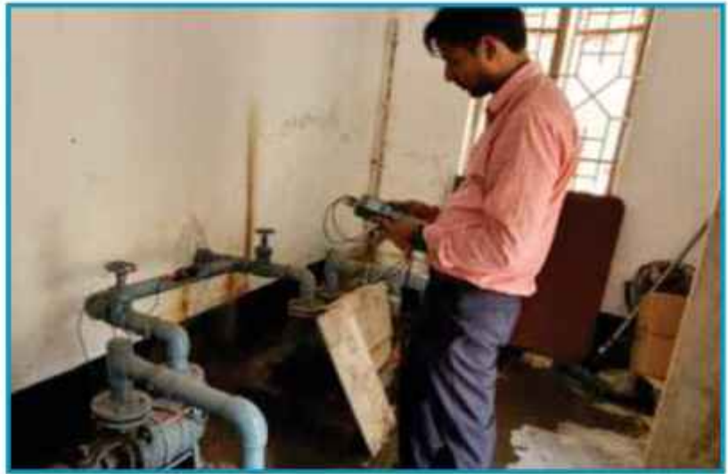
Monitoring & measurement for water audit by NPC team
